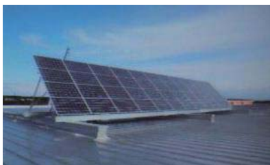
Solar panels on the school building
