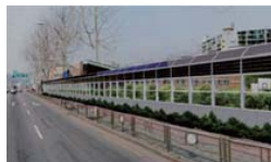
< PV on soundproof walls >
